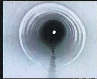
The proprietary EcoCast system applies the structural geopolymer with a high level of efficiency and precision
