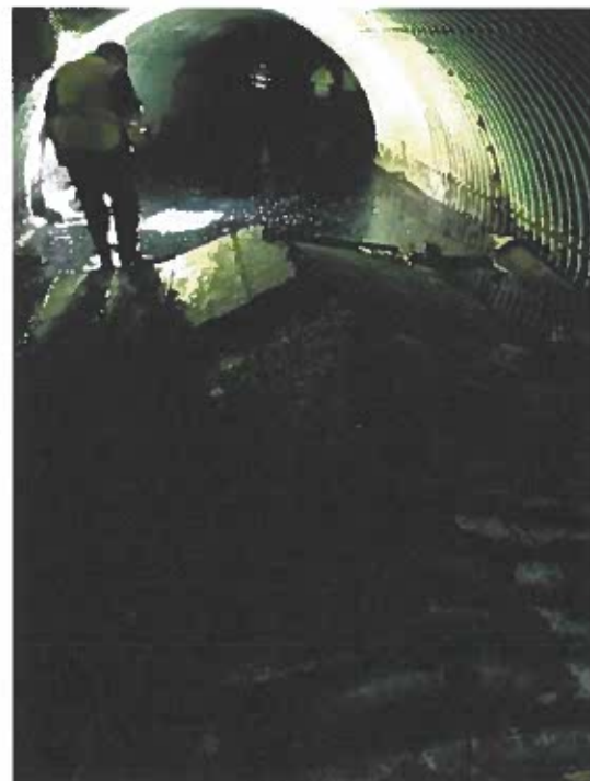
Figure 6 Second Upheaval Section, Arch CMP and Concrete Floor Heaved
