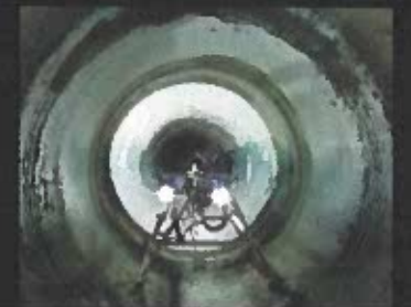
Concrete, sanitary and storm sewers
