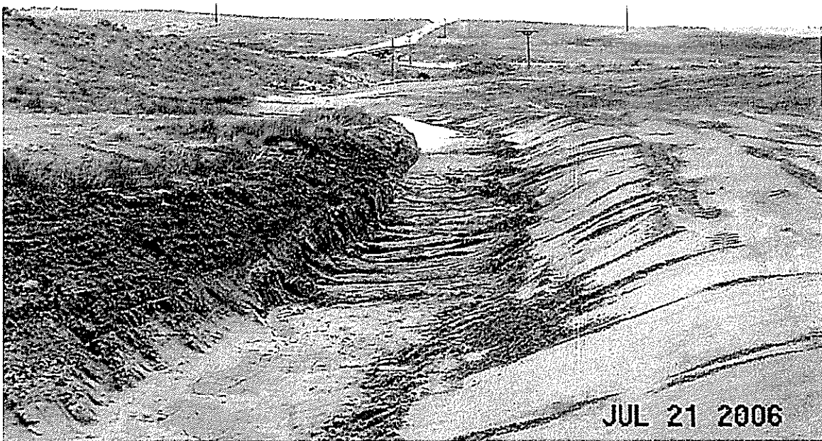
Space Village, 28" CMP, Outlet Channel in Fair Condition. Appears to be drainage.
