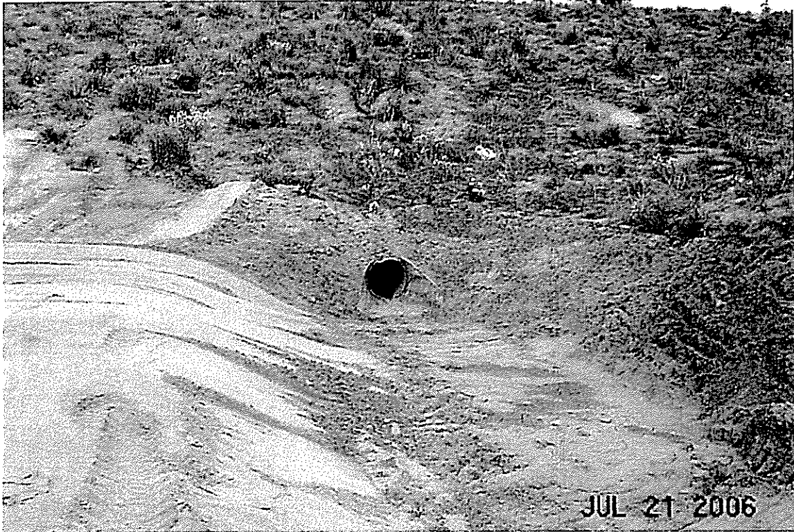
Space Village, 28" CMP Outlet, bent.
