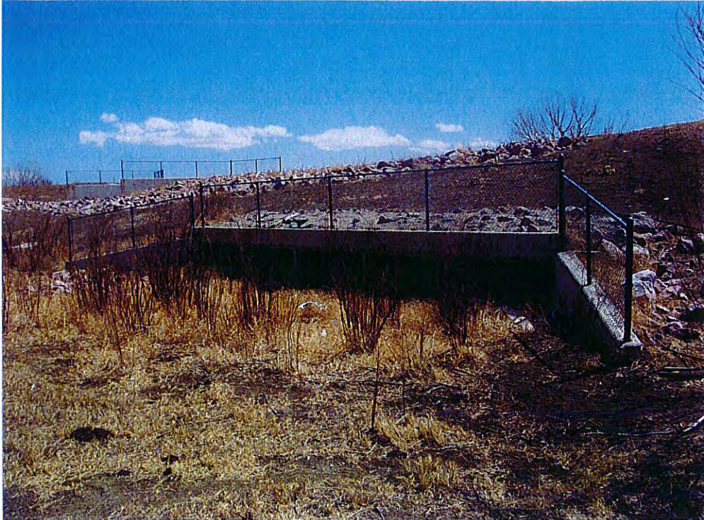
Existing (5) cell box culvert outfall. Each cell measures 6' wide by 3' tall. Invert is at elevation 5746.50.
