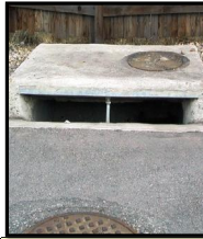
Denver No. 14 Curb Opening
