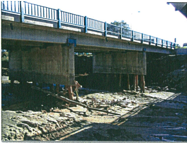
Photo 3-Damage to Platte Bridge
