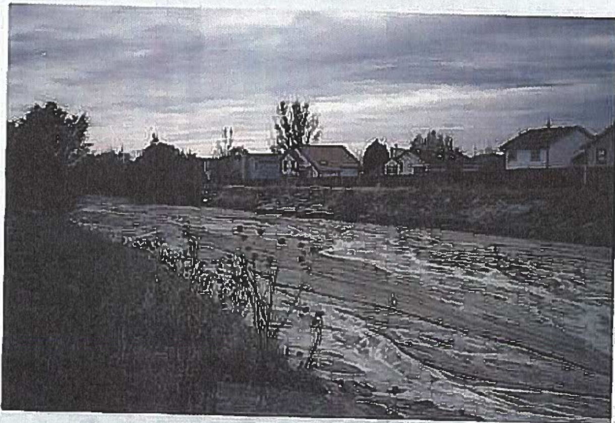
Sand Creek - 11/3/97 +/-Sta. 183+00 Eroded Grouted Rip-Rap Looking West from East Bank
