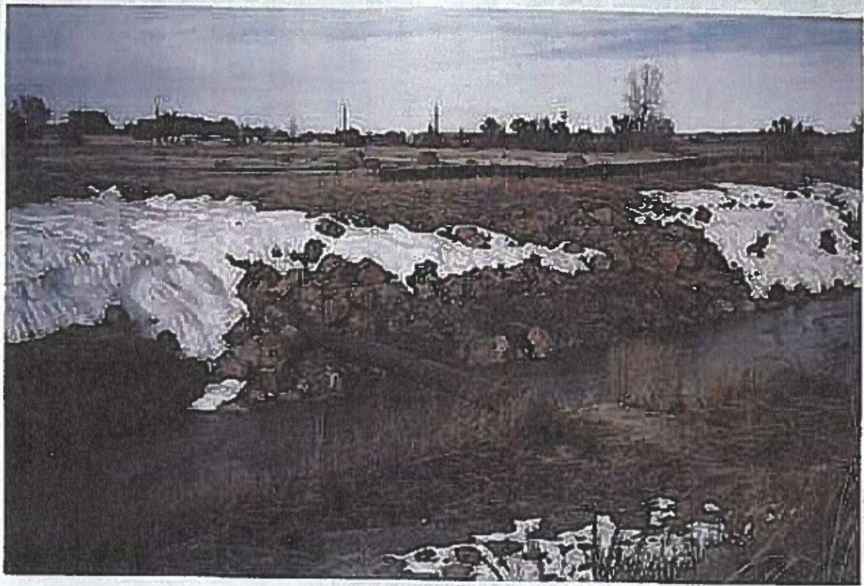
East Fork, Sand Creek - 11/3/97 Existing Conduit Sta. 43+00+/- Looking North from South Bank
