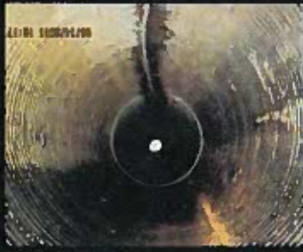
Typical condition of a corrugated metal pipe in need of repair.
