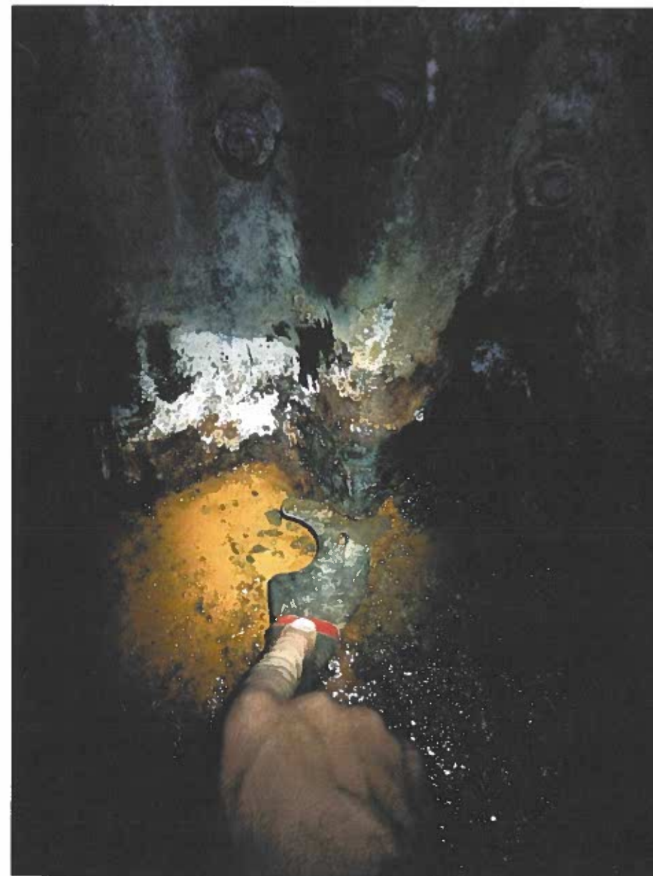
Figure 5-2: Through wall corrosion at the bottom of the culvert near the concrete floor.
