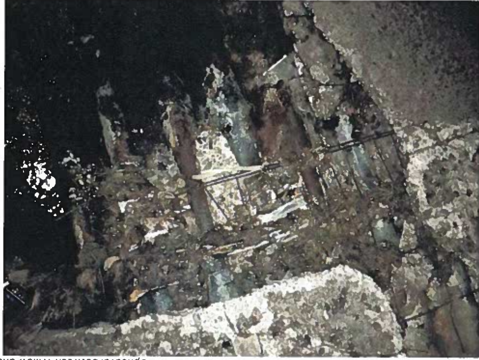
Figure 3 Upheaval between Willow and Hancock
