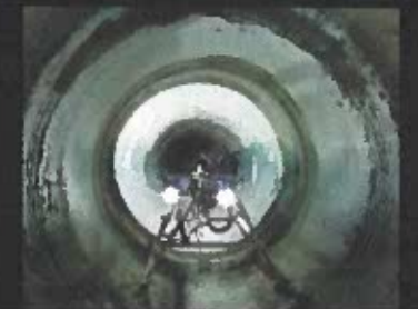
Concrete, sanitary and storm sewers
