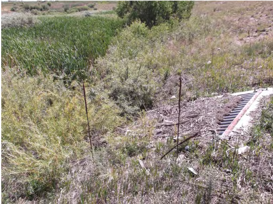
Photo2. Existing pond outlet with steel trash rack. Outlet consists of a 48" RCP with headwall and wingwalls. Constructed wetland is in the background and new wetland has established near the pond outlet.
