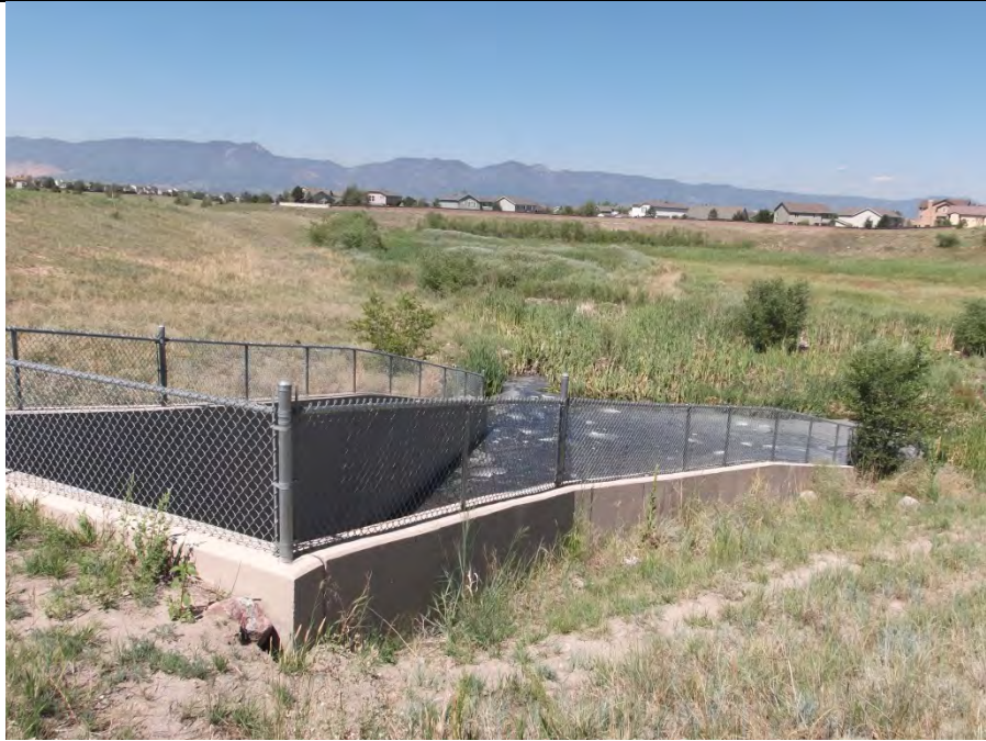
Photo 1. Looking west from main inlet culvert to RDF-C showing existing constructed wetland along south side of pond (left edge of pond bottom). Pond forebay is in foreground below culvert apron. Outlet is in the distance in the southwest corner (top left area of photo).
